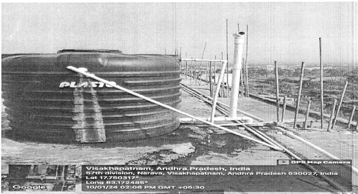
Waste Water Recycling in boys Hostel
